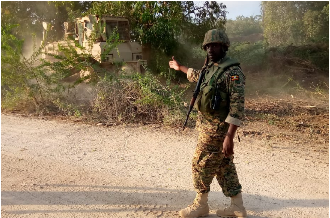
An ATMIS Uganda soldier directing ATMIS road construction machine clearing bushes along the Buufow-Janaale main supply route in Somalia on 25 February 2023.
