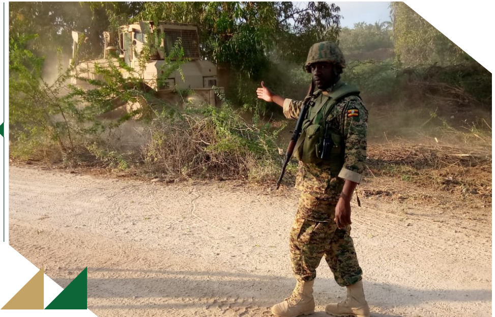
An ATMIS Uganda soldier directing ATMIS road construction machine clearing bushes along the Buufow-Janaale main supply route in Somalia. - 25 February, 2023.
