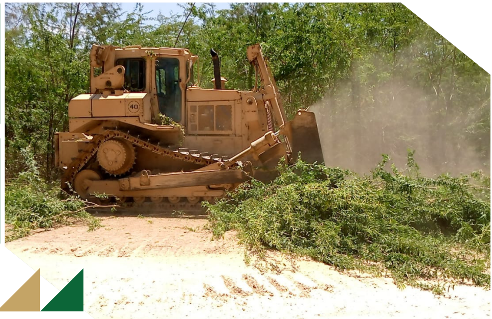
An ATMS earth moving machine clears thick bushes along the Buufow-Janaale main supply route in Somalia. - 25 February, 2023.
